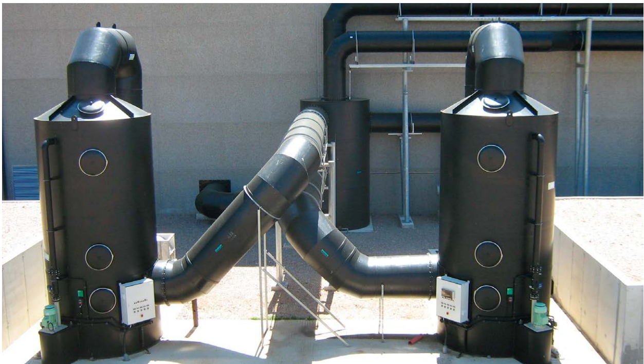
Immersible pumps on scrubbers
