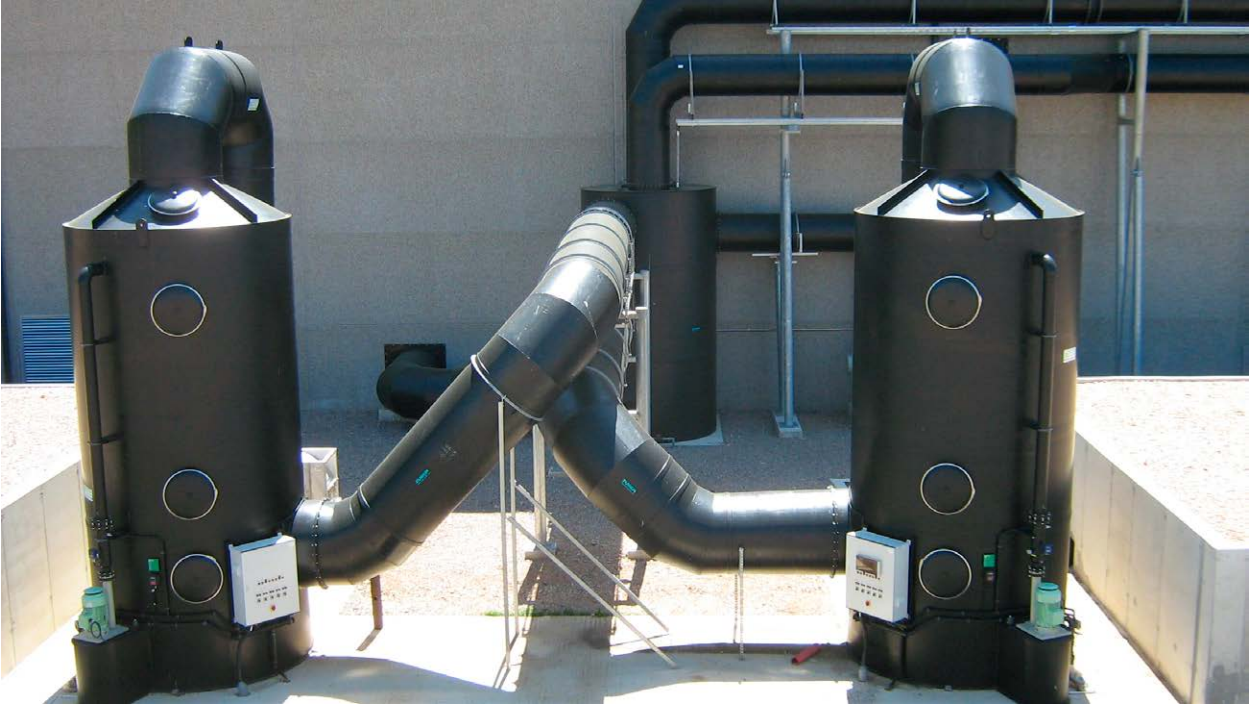
Immersible pumps on scrubbers
